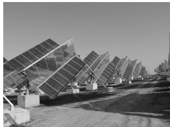
Fig. 3. – The tracking ridge concentrators with bifacial PV panels (0.5 MW p PV power plant)
