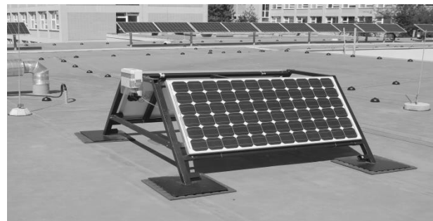
Fig. 1. – Frame with panels installed on the roof – situation
